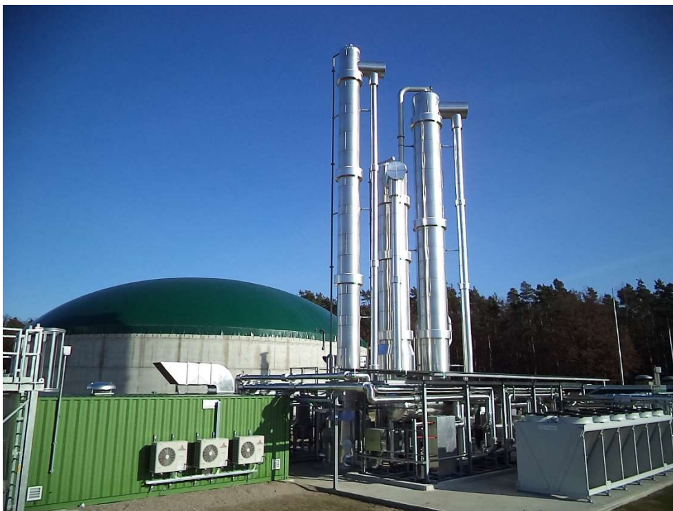
Figure 8. Organic physical scrubber from BMF Haase in Wolfshagen, Germany
