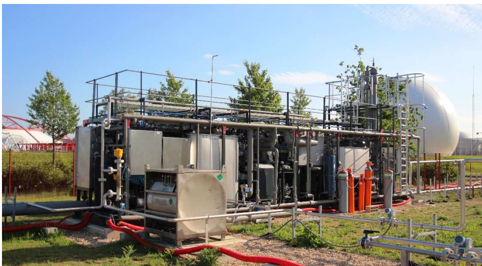
Figure 11 Cryogenic biogas upgrading and liquefaction, pilot plant from Cryo Pur, Valetton, France
