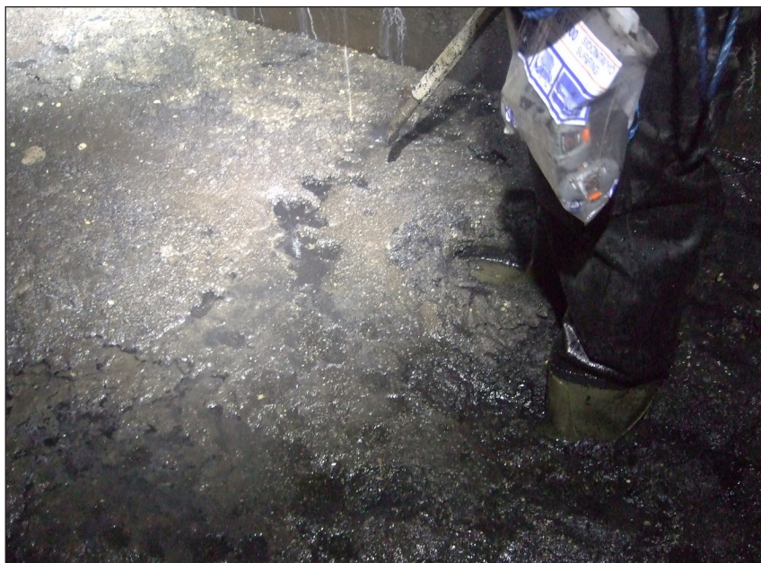
Figur 6-6 Slam/sediment i Sicklatunneln, Nacka (Mats Wåhlin AB, 2009).
